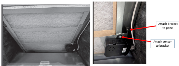
Figure 25: First A2L Sensor Mounting and Placement
