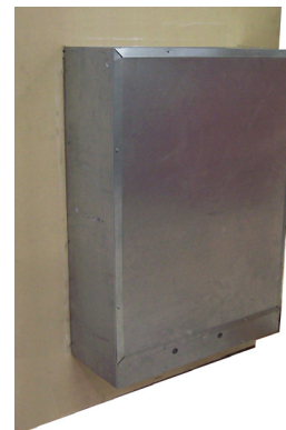
Figure 2 Shown with Insulation Jacket Installed
