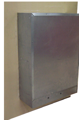
Figure 2 Shown with Insulation Jacket Installed
